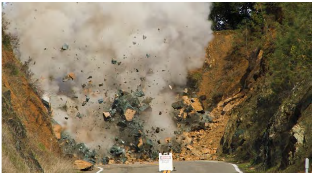
Blasting on Old Foresthill Road to clear rockslide caused by 2023-24 winter storms
